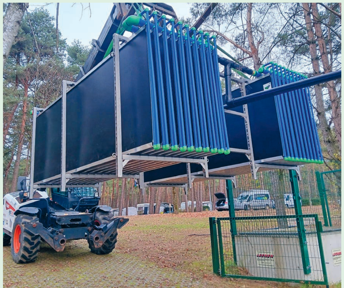
In December 2025, the heat exchanger was installed in the swimming lake at Camping De Lilse Bergen.
